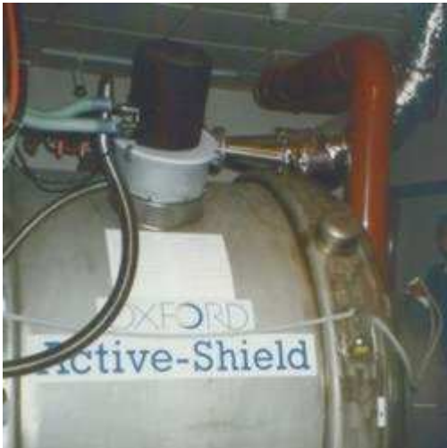
Typical MRI magnet shield
